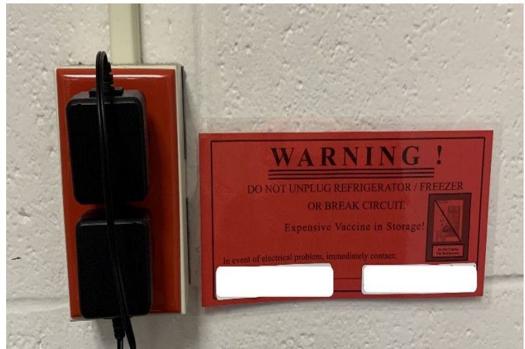
Example of a labeled outlet
