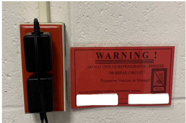
Example of a labeled outlet
